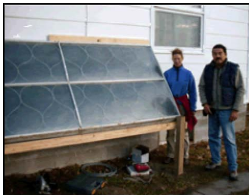
Solar Air Heater for House on Pine Ridge Reservation
